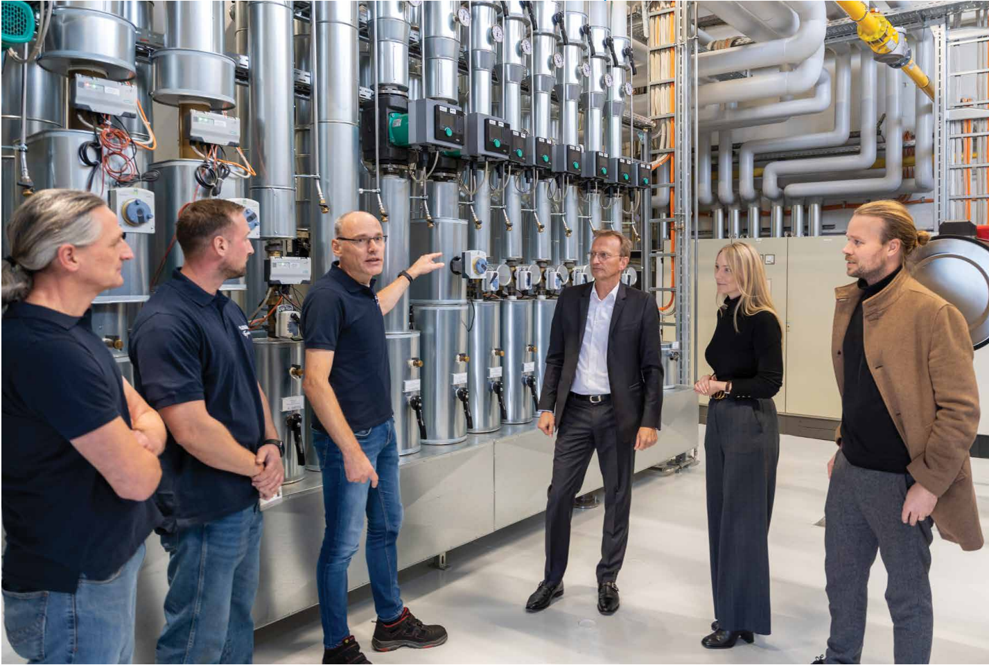
+ Project manager Robert Iding (3rd from left) explains at the new heating distributor how the waste heat from the hardening shop is fed into the Flender buildings. Also present: company electrician Roger Hogefeld and plant mechanic Philipp Holtmann (left) as well as Flender CEO Andreas Evertz, Head of CSR Kimberley ten Broeke and Head of Flender Real Estate NRW Markus Ritte (right).
